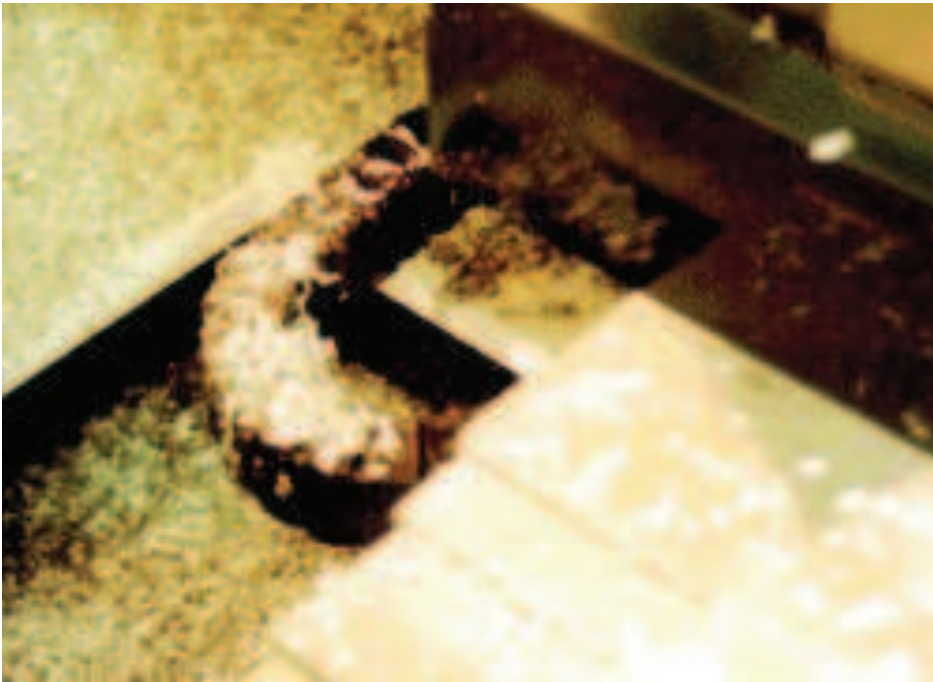
E2 E-Tubes side-mounted and unsupported in a chip area
